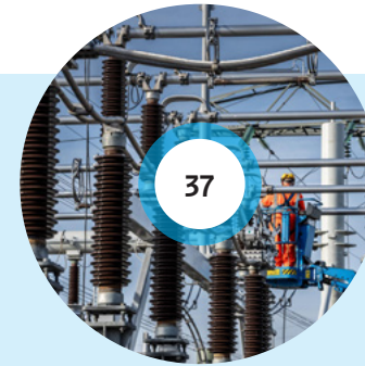
380/150 kV-station Port of Moerdijk
