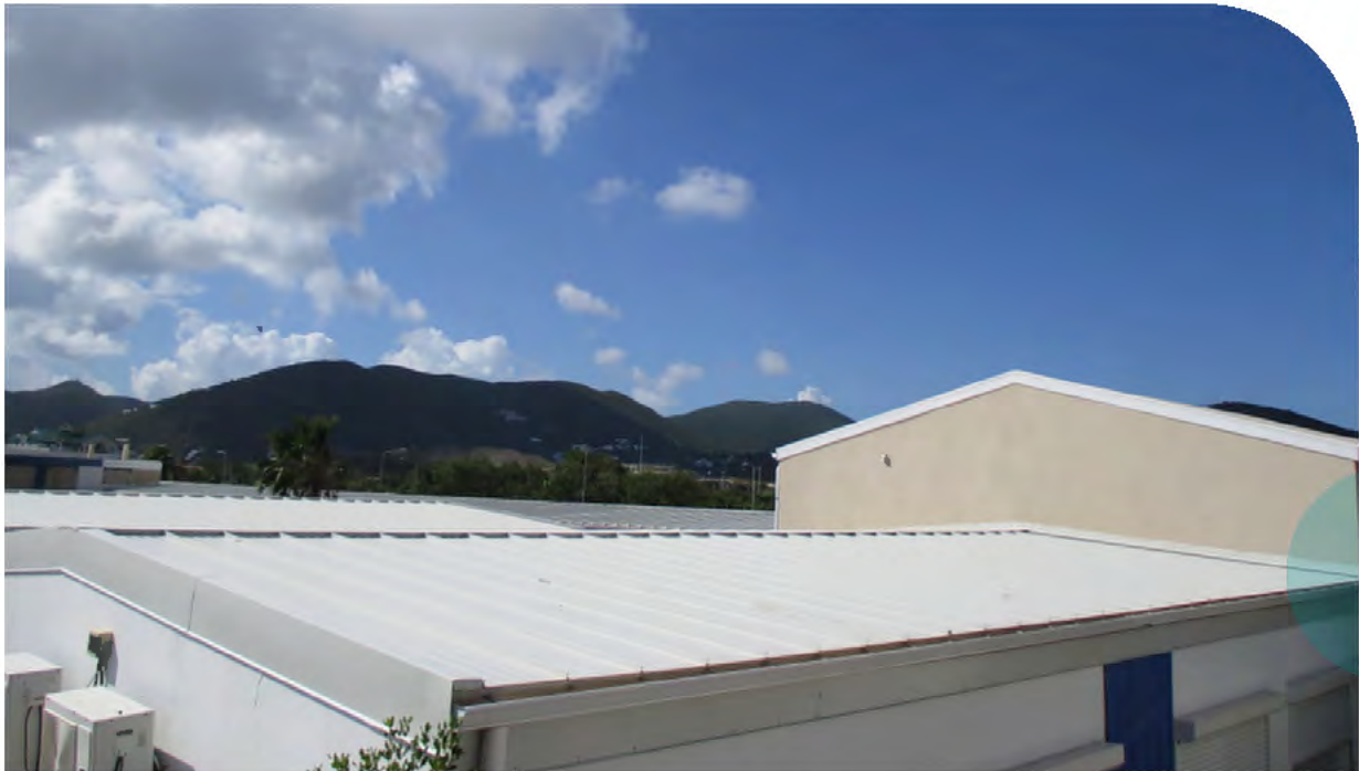
Nineteen school structures have been repaired and structurally refitted, creating a safer environment for students and staff post-Hurricane Irma, and strengthening resilience to future hurricanes. (Photo credit: NRPB)
