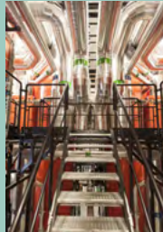
Combustion systems of bio heat power plant 'De purmer' (p 11)
