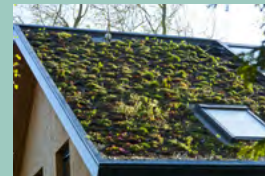
A green roof is an eco-friendly form of insulation (p 24)
