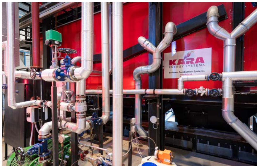
Biomassacentrale in Lochem.
