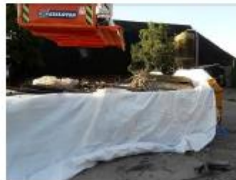
Foto: asbest in container
