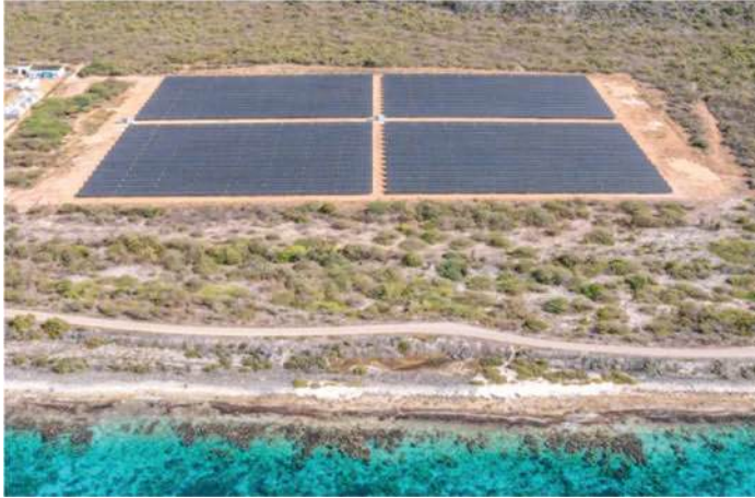
Figure 4.1 Bonaire solar park. Source: The Green World Company
