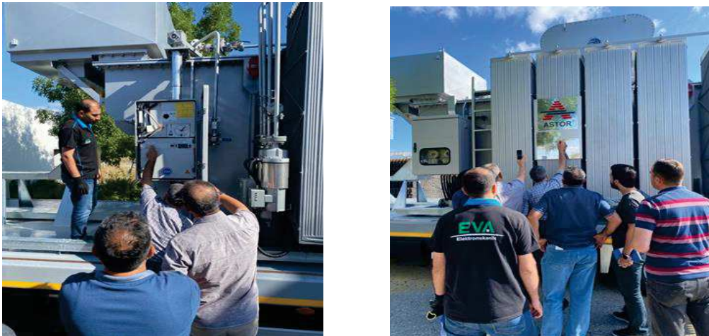
Engineers are testing the tap changer tests (left) and are verifying the specifications and name plate of the substation (right).
