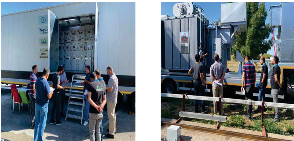
Visual inspections of the switchgear cabinet (left) and tap changer (right) were carried out.
